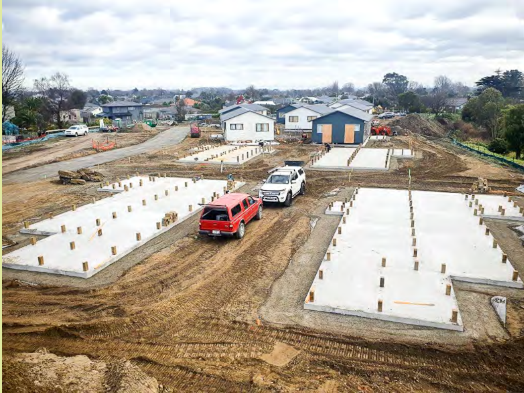
Foundations being laid at the former Churchill site, Guild St for 15 social housing units
